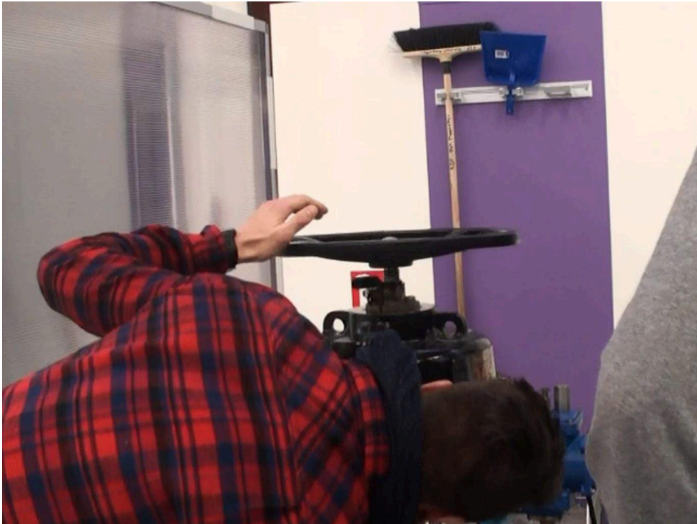
Figure 16 : Stagiaire observant la tige de la vanne lors de son ouverture. Figure 16: Trainee views the valve stem as it opens
